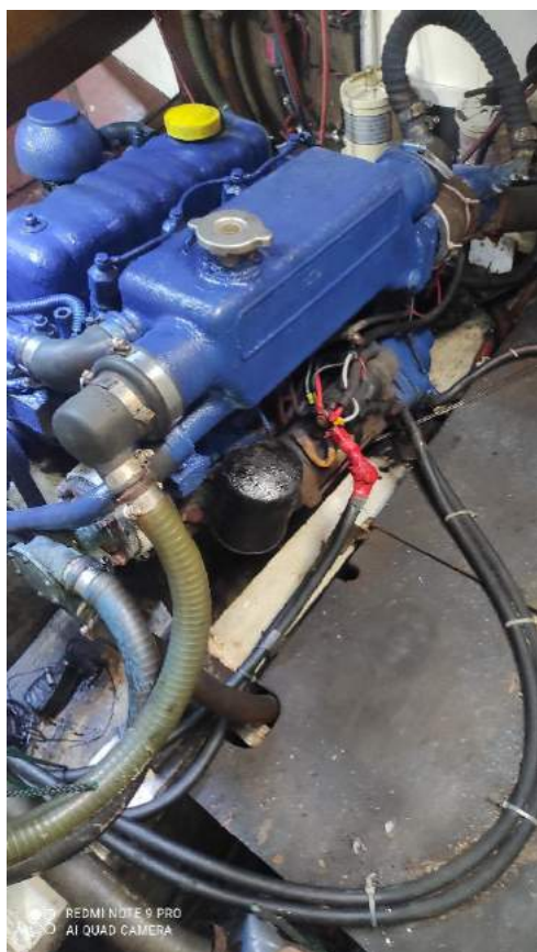
66_engine_port_side_oilfilter_starter heat exchanger and raw water pump
